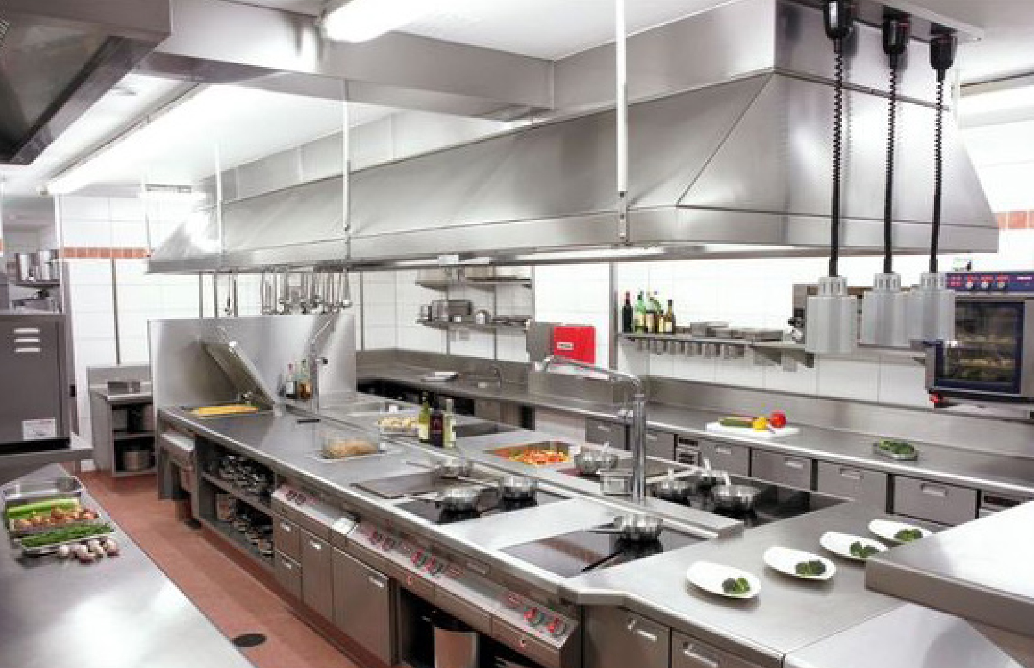
xxxx sq.ft. back of house kitchen serving IRD, employees and F&B outlets. Banquet kitchen near meeting rooms. TBD by Kitchen Consultant and Ops.
